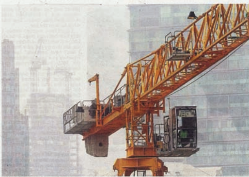
Going up: A tower crane at a construction site in Kuala Lumpur in this file picture. Operators must have valid certificates of competency from DOSH.
