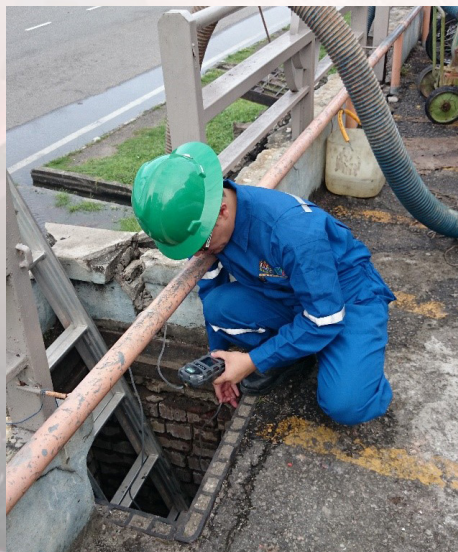
Figure: 'Atmospheric Testing before Entry' being conducted by an Authorised Gas Tester.
