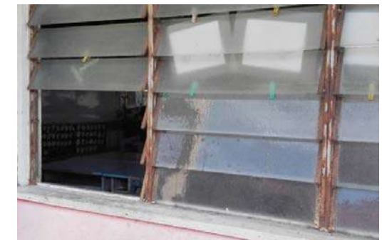
Figure 8: Rusted window glass holder
