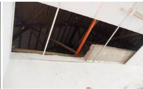
Figure 10: Ceiling tiles missing
