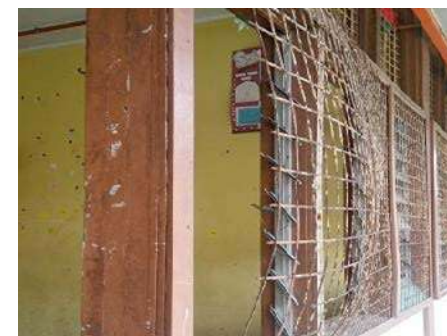
Figure 7: Broken window grill
