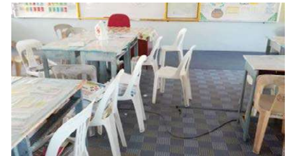
Figure 4: Electrical wire may contribute to slip, trip and fall
