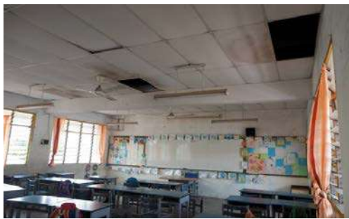
Figure 9: Ceiling poorly maintained and molded
